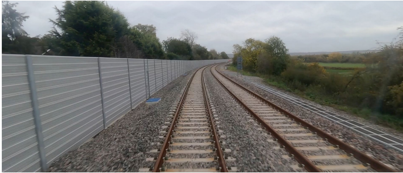
Figure 15: Photograph of an existing noise barrier installed between Bicester and Bletchley
